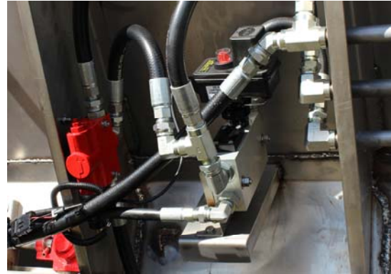
Hydraulic control valves for conveyor and spinner control
